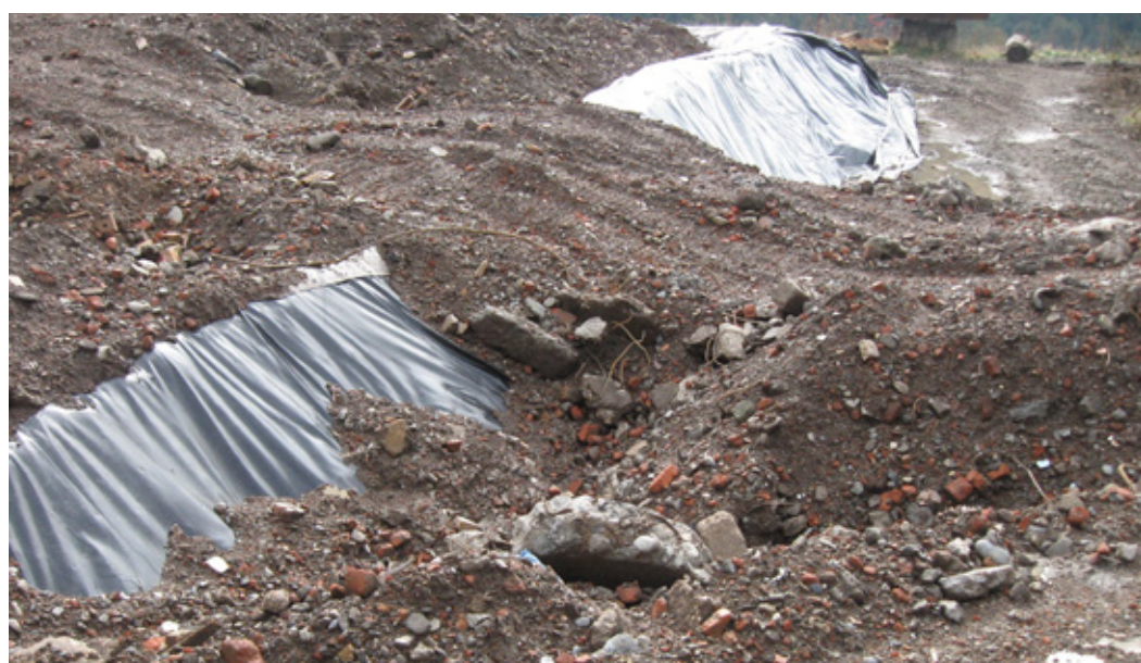
Figure 4 - The presence of sharp/big stones without protective geotextiles will significantly increase the risk on damaging the geomembrane [Gerritsen]
