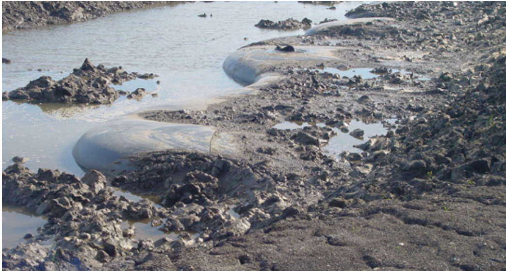
Figure 6 - Geomembrane 'whales' due to uplifting water pressure below the geomembrane related to improper backfilling levels [Genap]
